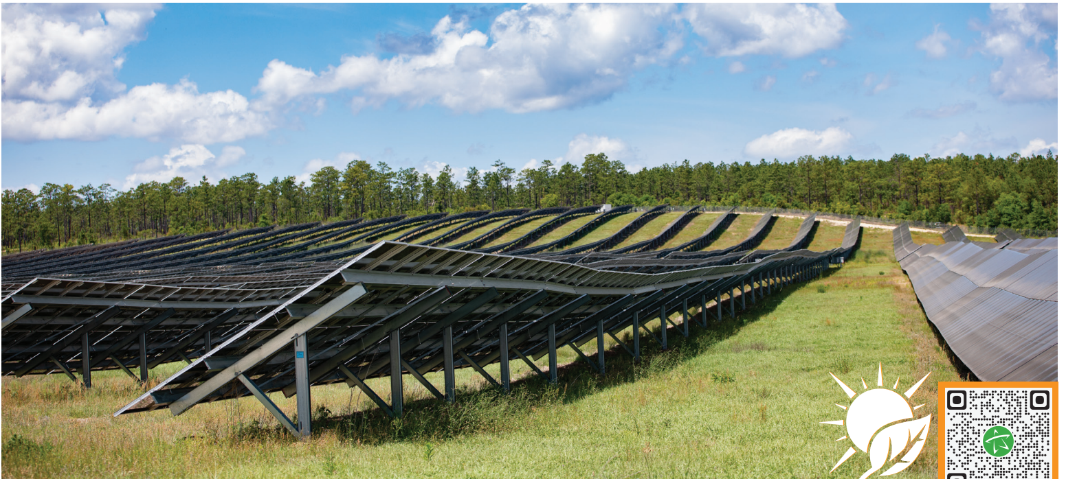
City of Tallahassee Solar Farm
