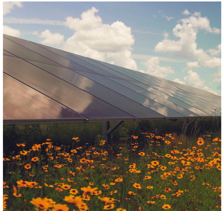
City of Tallahassee Solar Farm
